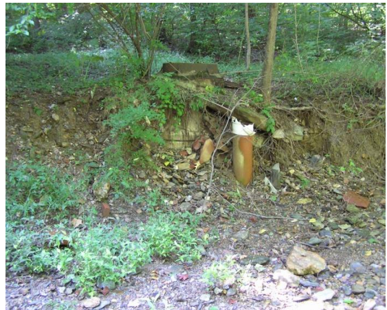
Erosion along sewerline
