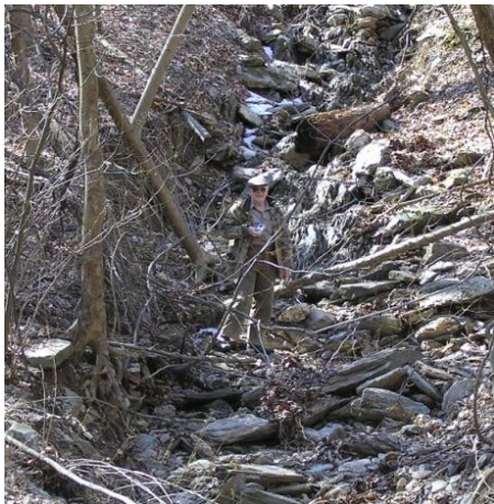
Erosion below storm water outfall (note person in center of photo)
