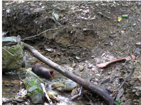
Broken lateral allowing surface water to get into sewer
