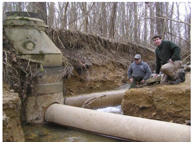
Headcut eroding under sewerline on Jan 15, 2005
