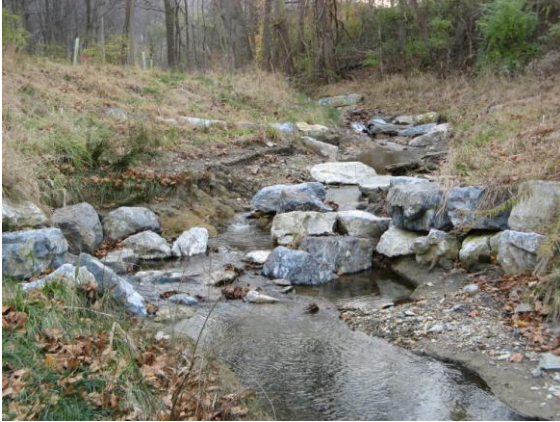
Failed structures in restoration due to erosion of underlying silt
