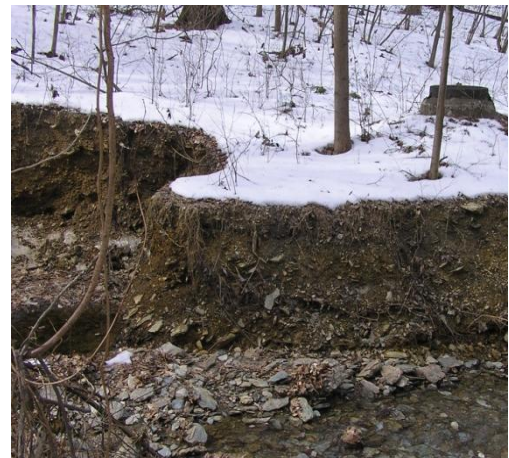
Erosion along sewer line above RR tunnel
