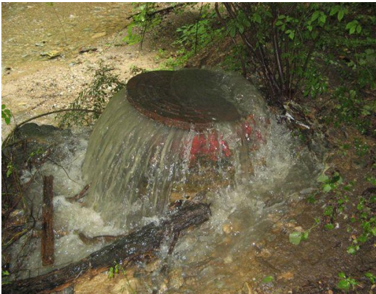
Sewage spouting from broken manhole cover above RR
